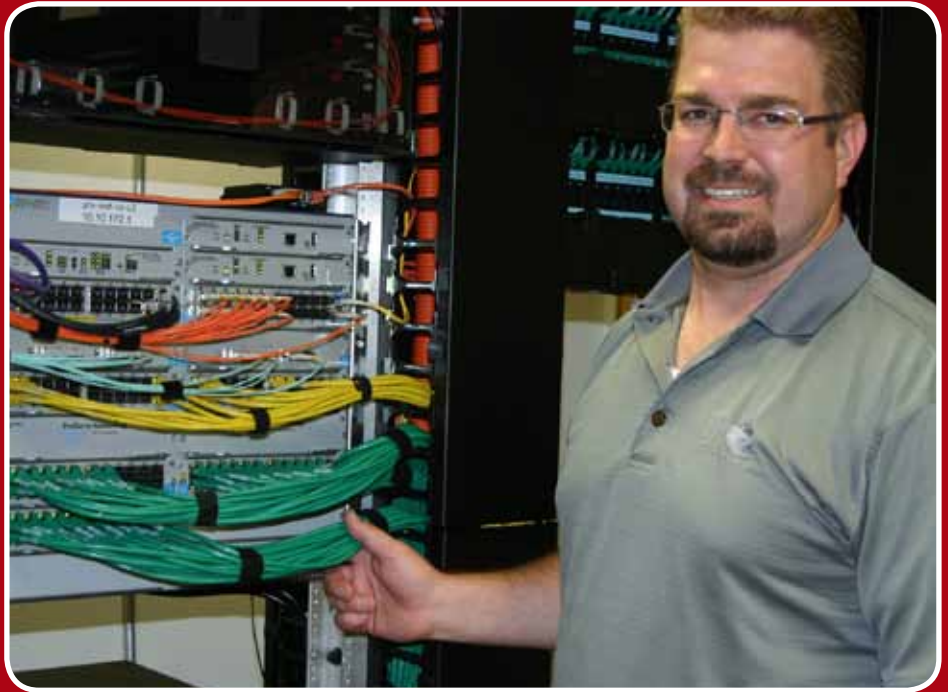
Chad Blotkamp with CTS in Tempe, Ariz. Checks out the patching of the new cable in one of Gilbert's high school's TR.
