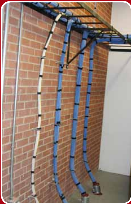
During expansion of Kingman High School, a wing was connected to the previous school, which required the TR to be located between the outer wall of the existing building and the new addition.
