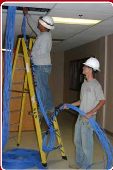
CTS installers Daryl Begay (on ladder) and Dillon Franssen install category 6 cable for the Gilbert School District.
