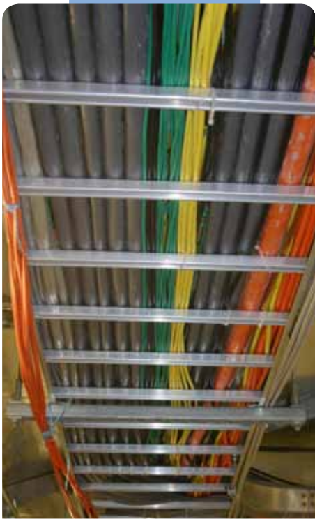
Cable pathways in a health care environment share space with other systems, such as HVAC, gasses and electrical services.
