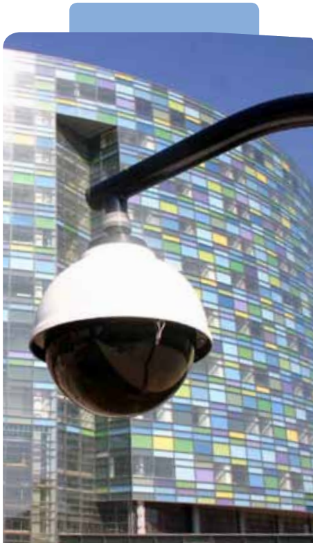
With IP convergence, many applications are running over one cable. Pictured here is an IP-based security camera running over Category 6 cable at Johns Hopkins Hospital.
