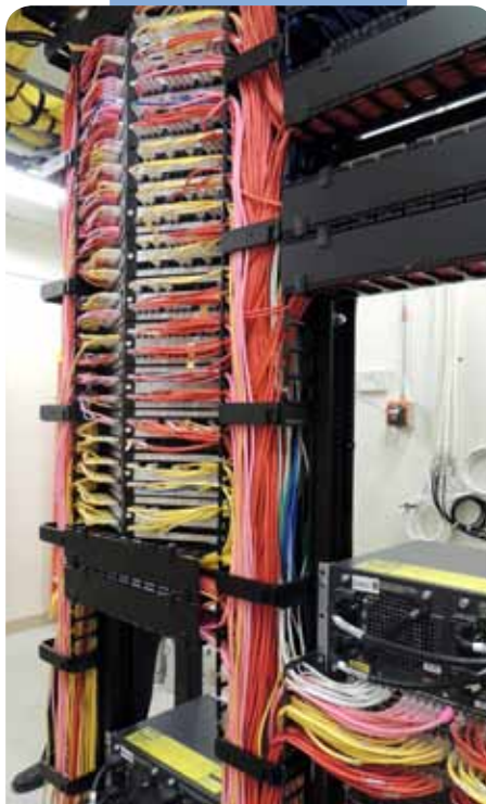
Because of the diverse applications in a health care facility, it is recommended that the cable be color coded and terminated to its dedicated active equipment.
