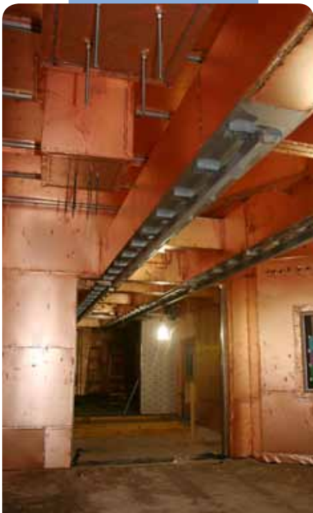
A special radiology unit at Johns Hopkins Hospital features copper-lined walls to act as an RF shield and optical fiber cable for resistance to electrical interference.
